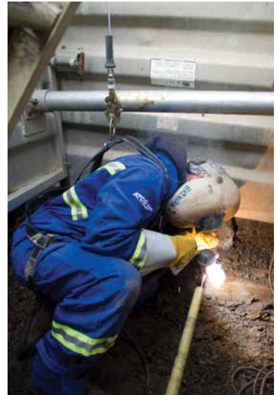
Brendan Walton, Pressure B Welder, ATCO Gas, uses an emergency trench rescue device while welding a stopper fitting onto a steel main. The device is used when employees are working in confined or restricted spaces enabling them to be quickly lifted to safety should the need arise.
