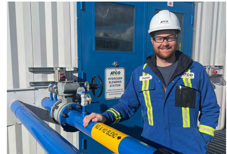
Our people are advancing innovative hydrogen projects to meet our customers' needs to reduce GHG intensity.
