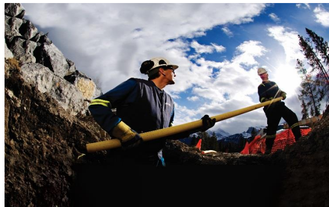
NATURAL GAS DISTRIBUTION $2.8B Rate Base
