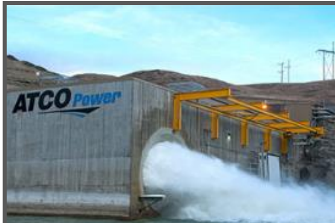
ELECTRICITY GENERATION CANADA 24 MW
