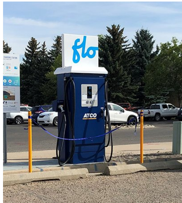
EV charging station, Lethbridge, Alberta
