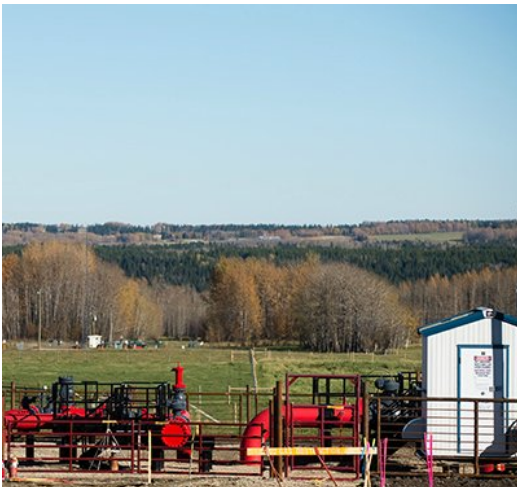
Natural gas transmission control station, Drayton Valley, Alberta
