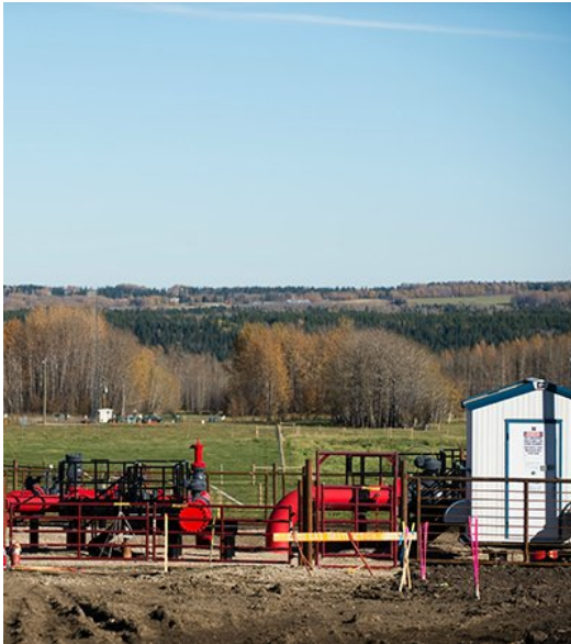
Natural gas transmission control station, Drayton Valley, Alberta
