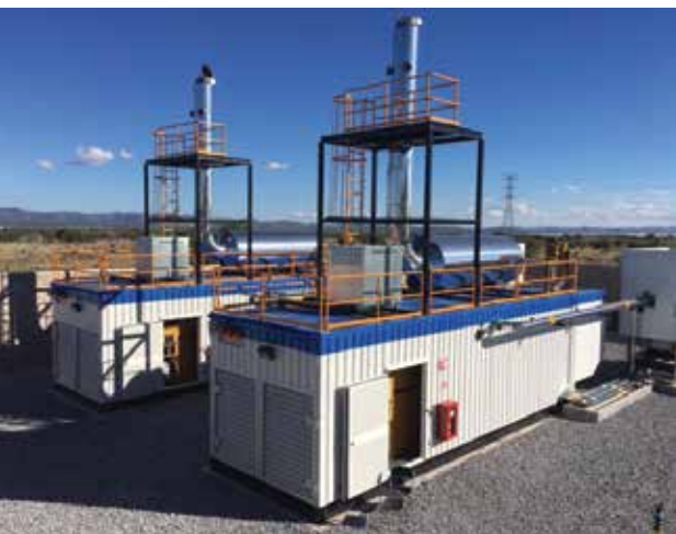
Our innovative distributed power generation solution will deliver up to 20 megawatts of reliable and efficient onsite electricity in a growing industrial park in Mexico.
