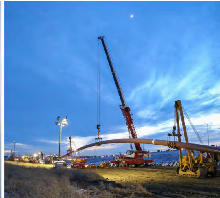
NATURAL GAS TRANSMISSION
